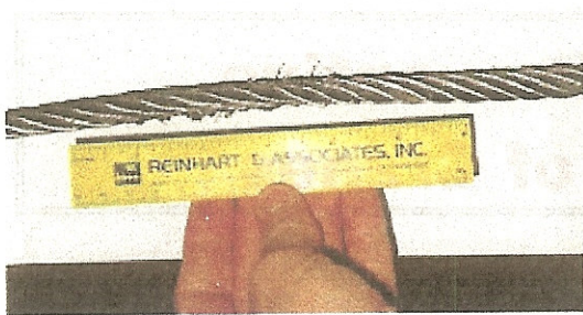
Damaged cable detected During crane inspection
