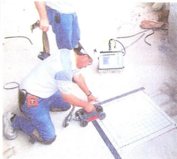
Reinhart & Associates, Inc. inspector scanning a concrete floor using GPR to locate rebar, cables and conduit prior to performing coring.
